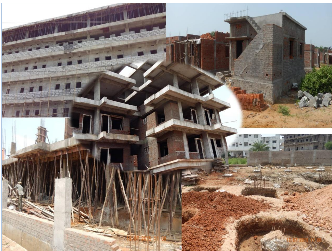
Figure 3-23: Under construction buildings provide insight into the construction materials and structural types
